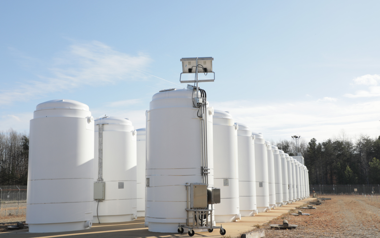
Dry storage systems and the High Burnup Research Cask at the North Anna Power Station.
